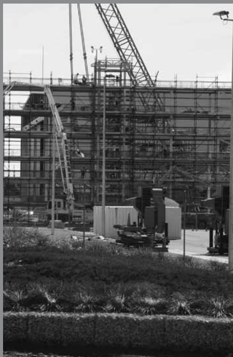
Support: The two Outfit Support Towers under construction will complete infrastructure requirements at ASC's shipyard (ASC South) to support the building of the Royal Australian Navy's air warfare destroyers.
