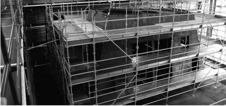
Ready: Block 715 ready for blast in the northern end of the main Blast and Paint Facility.
